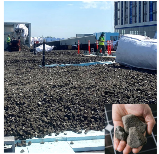
Capital One Center ‘The Perch’ Columbia Green Recycled Foam Glass Agg. Installation.
